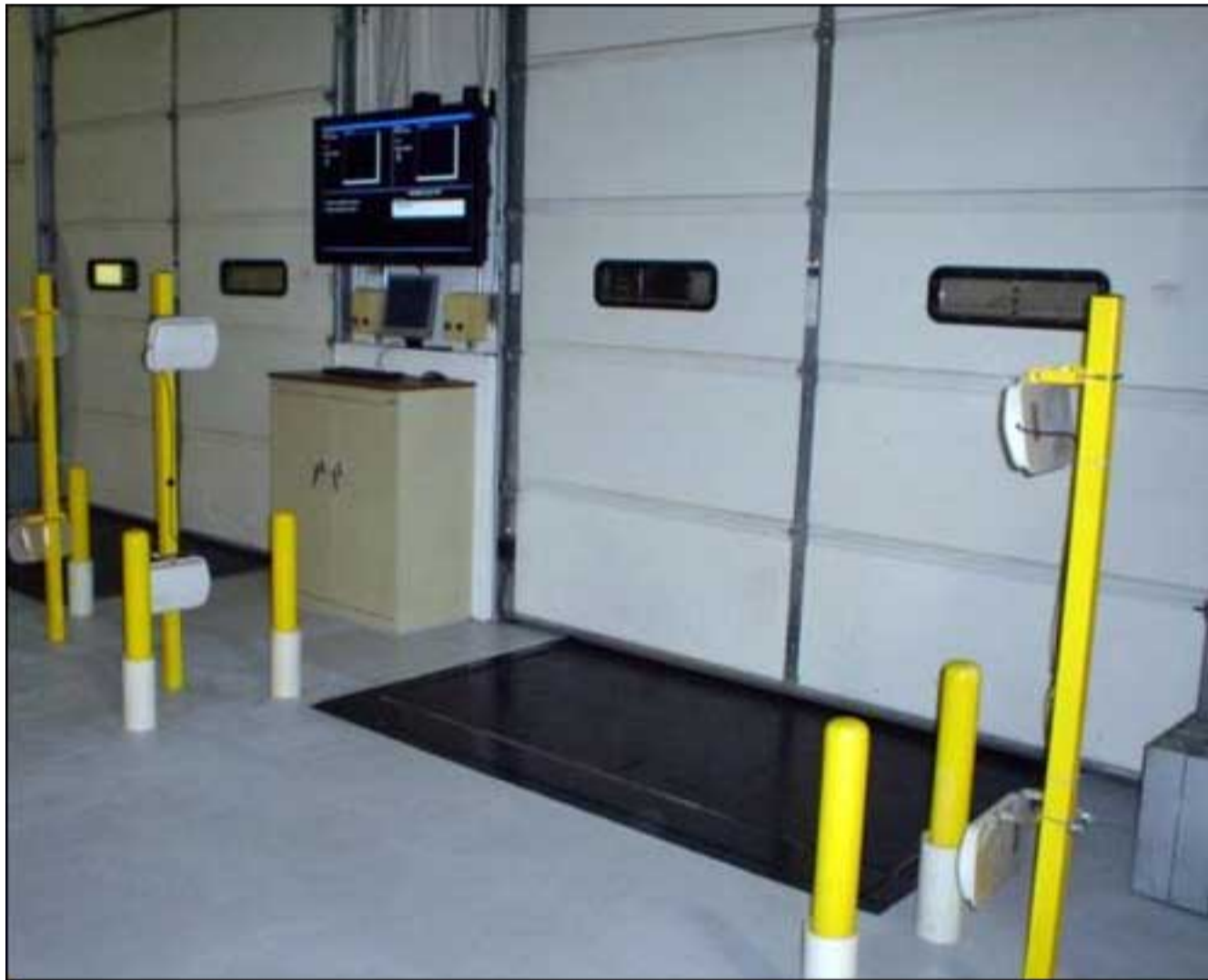
Color Point's RFID-enabled dock doors
